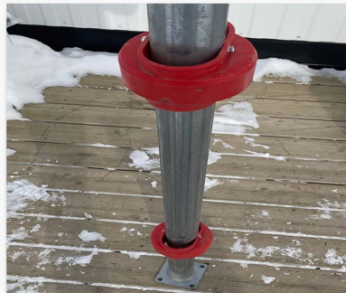
48" PIPE WITH BASEPLATE
